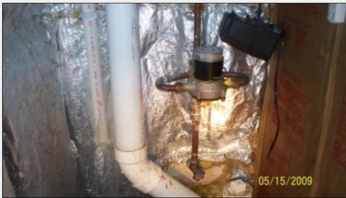
I-7: Leaking at valve
